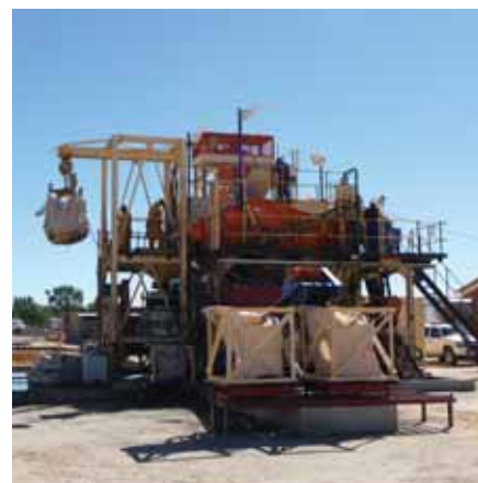
Tsabong Bulk Sampling Plant
